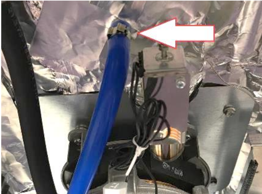
Figure 58. Steam generation tubes fastening
